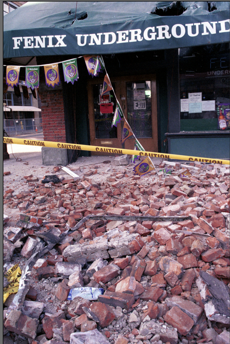
Seattle after the Nisqually Delta Earthquake, 2001 Photo courtesy of FEMA
